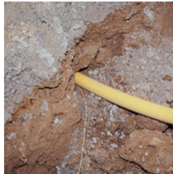
Underground Utility Locates (Potholing or Daylighting) Safely expose utilities without the threat of cutting or rupturing a line or pipe.
