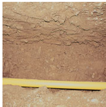
Trenching (New Trench or Exposure of Existing Lines) Cut trenches quickly and easily, or expose sections of lines, laterals and piping.
